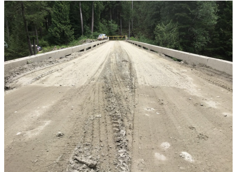
Sediment getting onto deck at right approach
