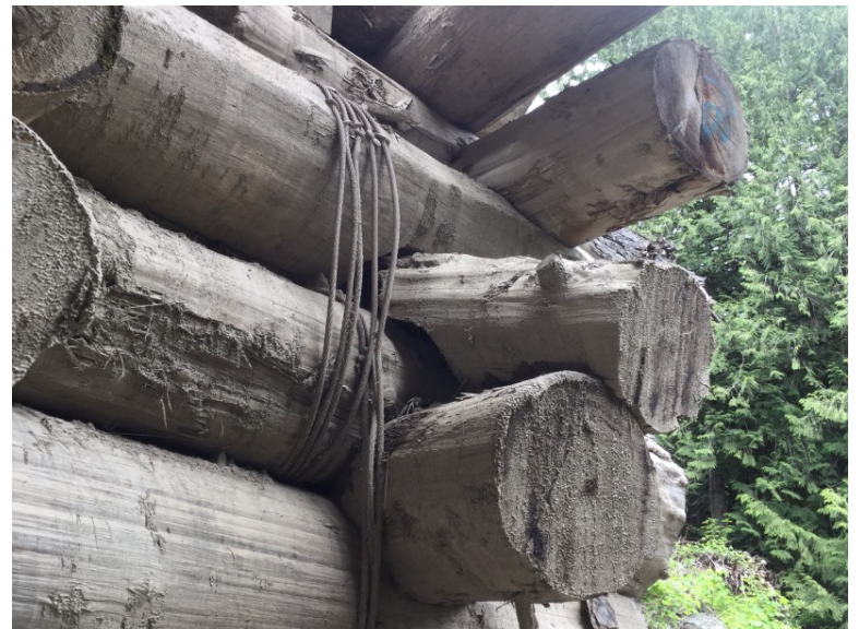
Broken tieback at upstream right bank
